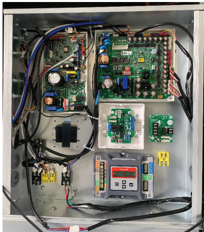
Split Rooftop Unit Relay Board
