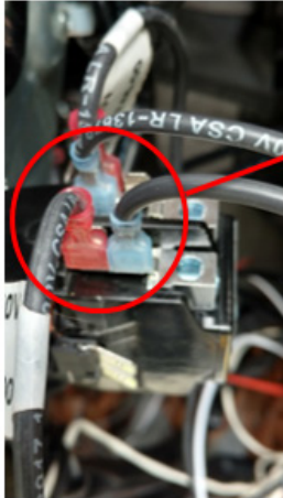
Contactor w/Heaters Connected Contactor Top View
